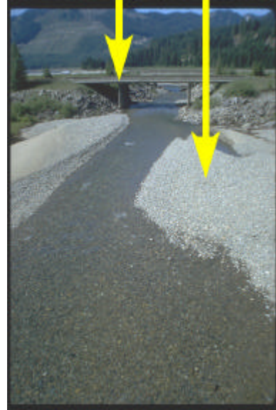
Poor Range (arrows emphasizing large-scale channel alterations)
